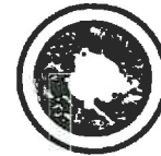
SINK OR DRAIN PIPE BUILDUP 30% FLOW
