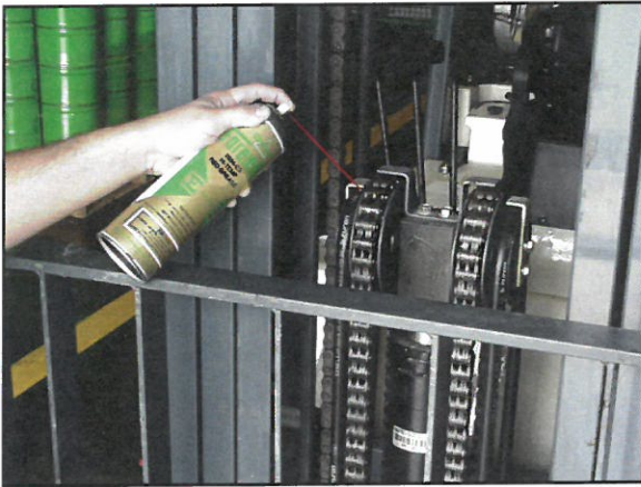
OPEN GEAR LUBRICATION
